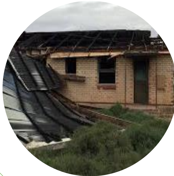
Roof Blown Off
