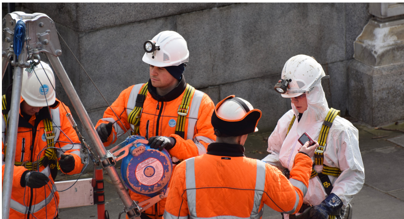
England's aging underground water mains pipe are prone to leakages without regular maintenance, making pipe leakages a priority for the water regulator Ofwat.
